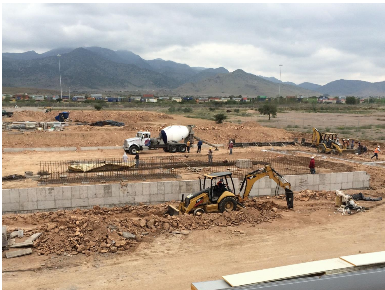
Solvay's new Technyl® compounding unit under construction in San Luis Potosí, Mexico. (Photo courtesy of Solvay)
